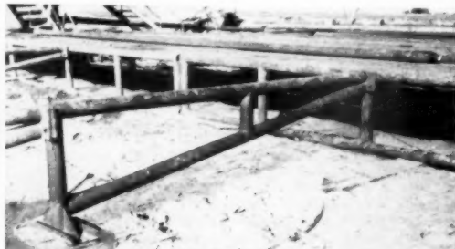
SUPPORT MEMBER. —View showing section of pipe-rack supporting member. Any one of these members may be used at any point.
